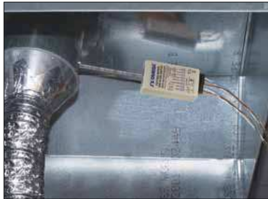
Measuring air flow and providing relay output in a ventilation hood.
