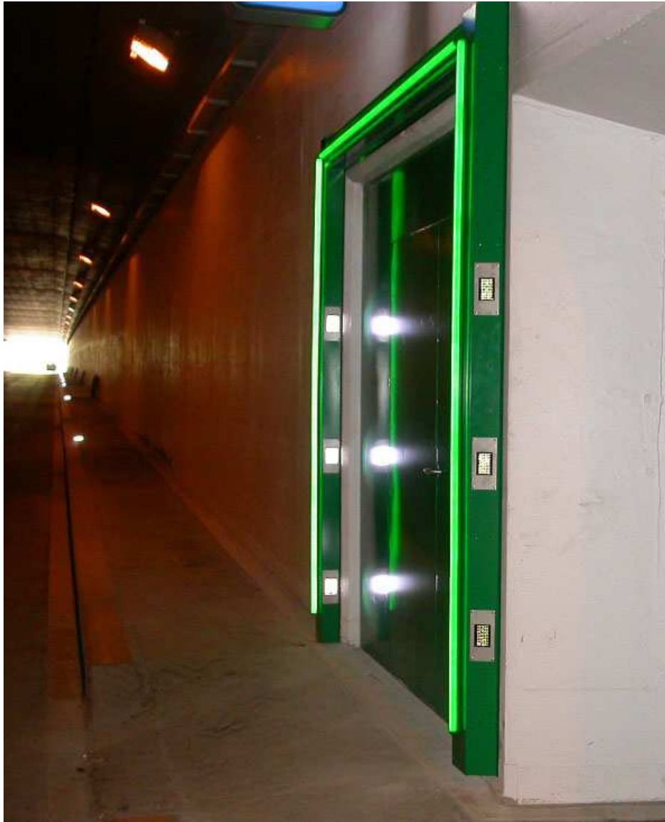
Emergency exit in road tunnel
