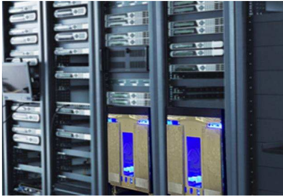
(2) TBYTe® Systems shown in Customer Racks
