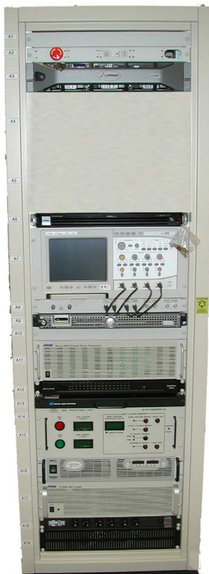
Example system rack configuration
